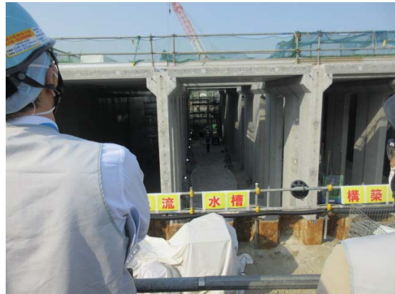
The dilution/discharge facility①
